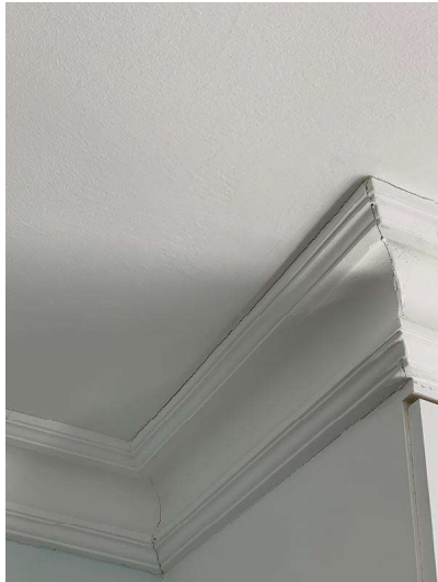
Photo 40 - Shrinkage cracking to coving
