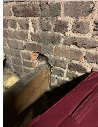
Photo 35 - Hole requiring filling
