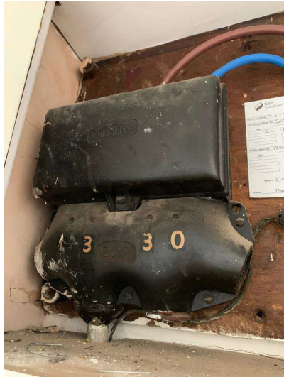
Photo 74 - Electricity head: possible asbestos
