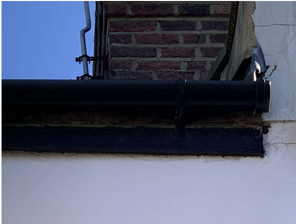
Photo 28 - Badly weathered fascia board
