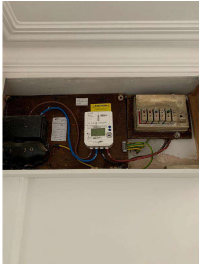
Photo 67 - Fuse board and electric meter
