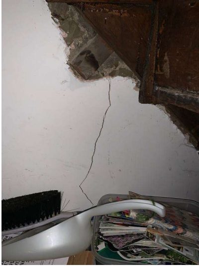
Photo 42 - Under stairs: large crack
