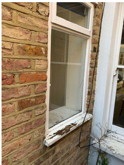
Photo 24 - Poor quality window with rotted sill
