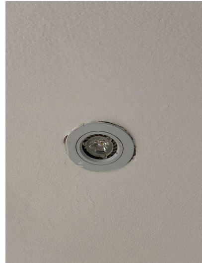
Photo 41 - Poor finish around spotlights
