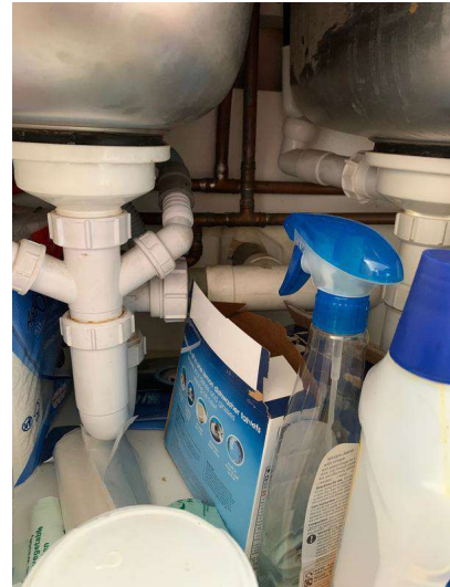
Photo 70 - Pipework under the sink
