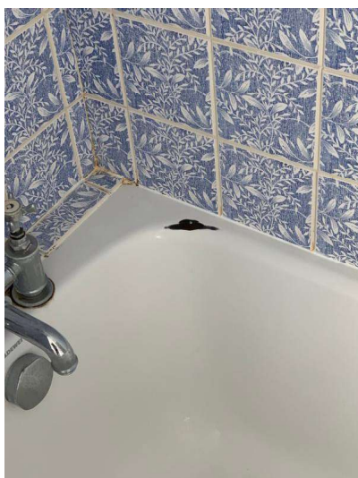
Photo 59 - Damage to bath
