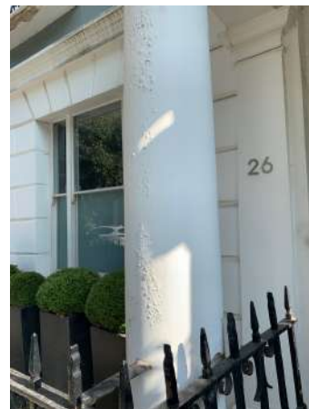
Photo 16 - Damp affected render to columns
