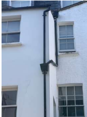
Photo 8 - Plastic rainwater goods
