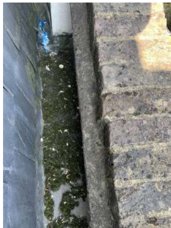
Photo 12 - Debris in box gutter
